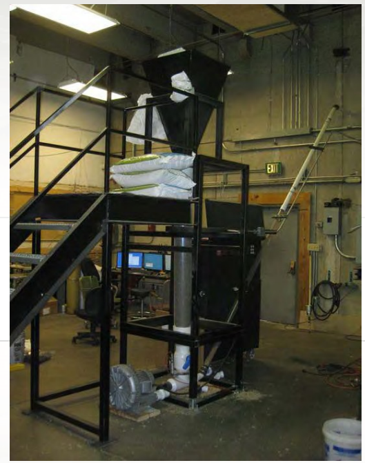
Pneumatic Conveyance System
